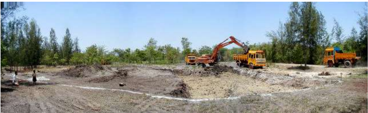
Tomas and Usha watch the excavator remove the black soil layer from the pond site
